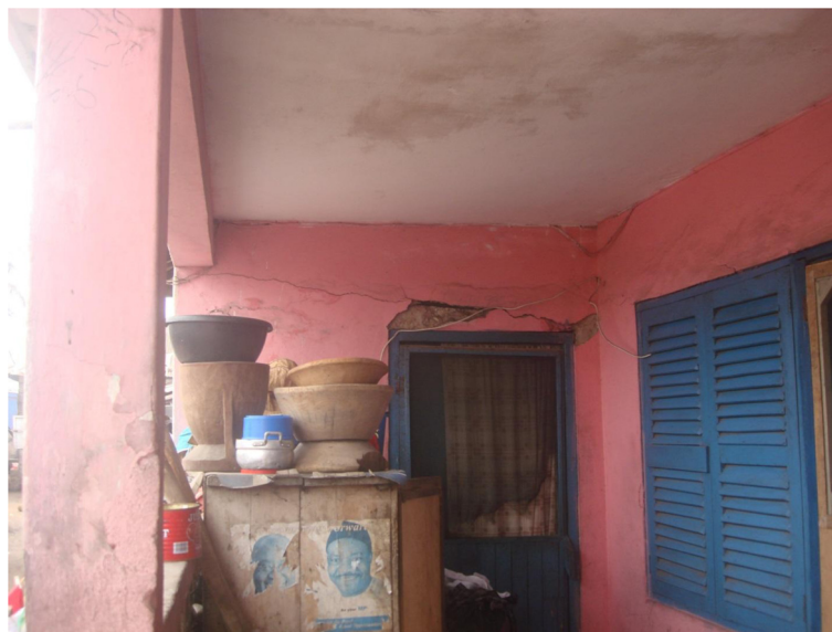
Figure 6 One of the houses in poor repair status. The house has cracks in the walls, a torn door net, and electrical wiring hanging off the walls.
