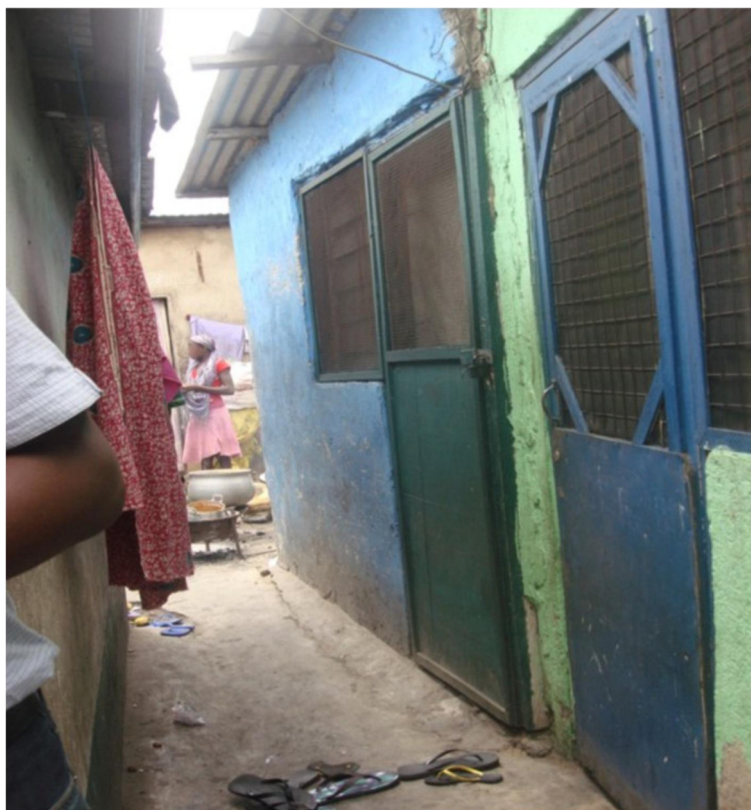
Figure 2 A multi-tenement structure in an informal settlement. Single windows on only one side of the building result in poor ventilation. Single rooms are occupied by families and lack privacy.
