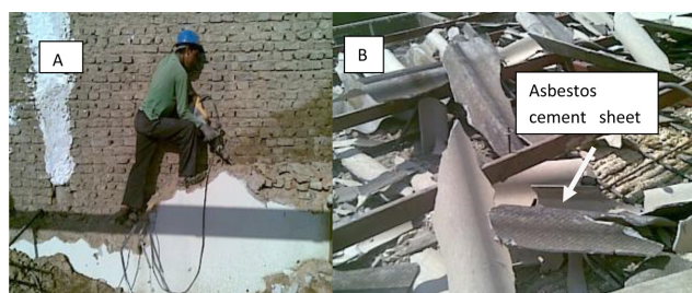
Fig. 1. Demolition in progress. (A) during demolition; (B) after demolition and before debris removal.
