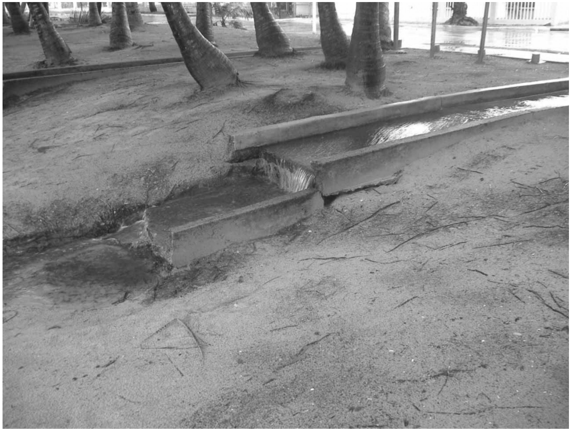
Figure 2. Outflow from main culvert draining storm water from residential area into transect 5 of the study area.
