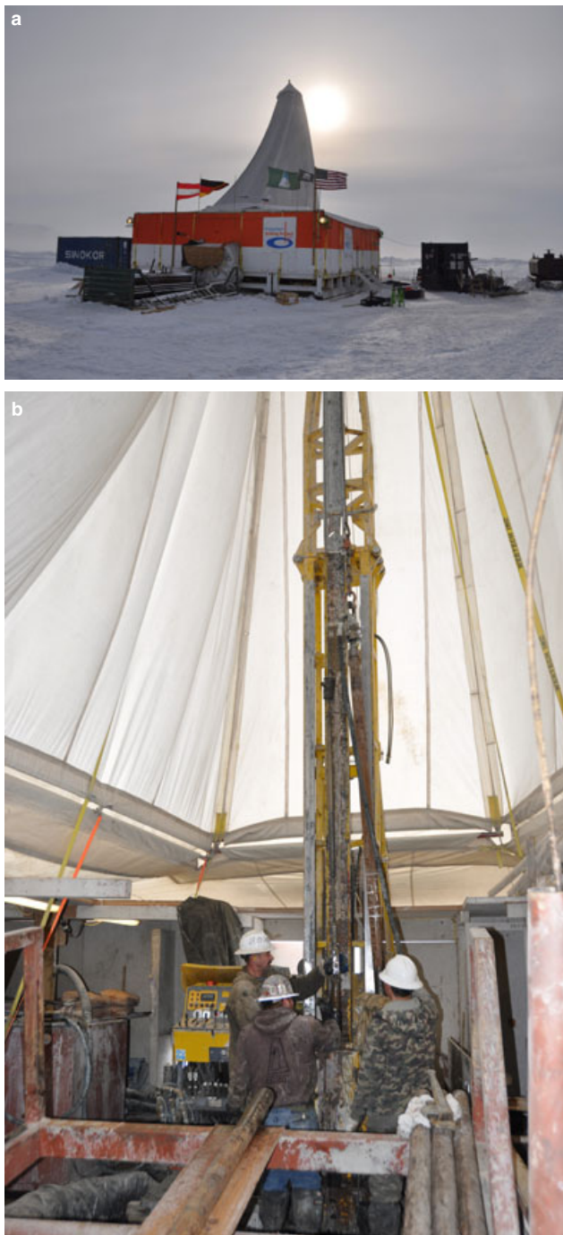
Fig. 7. a) The modified GLAD 800 drill rig on a platform contained within a tent to keep the interior above freezing, at ICDP Site 5011-1 at the center of the frozen Lake El'gygytgyn. b) The drill rig in operation within the tent.
