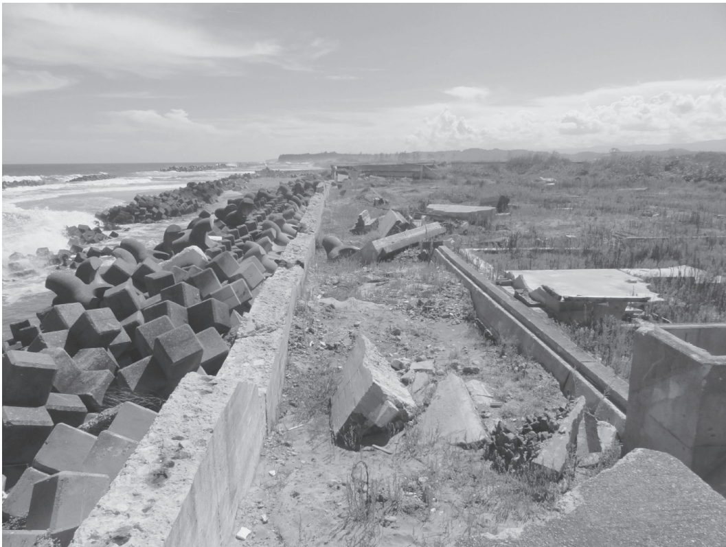
Fig. 6. Seawall destruction in Tsukabara (September 3, 2012).
