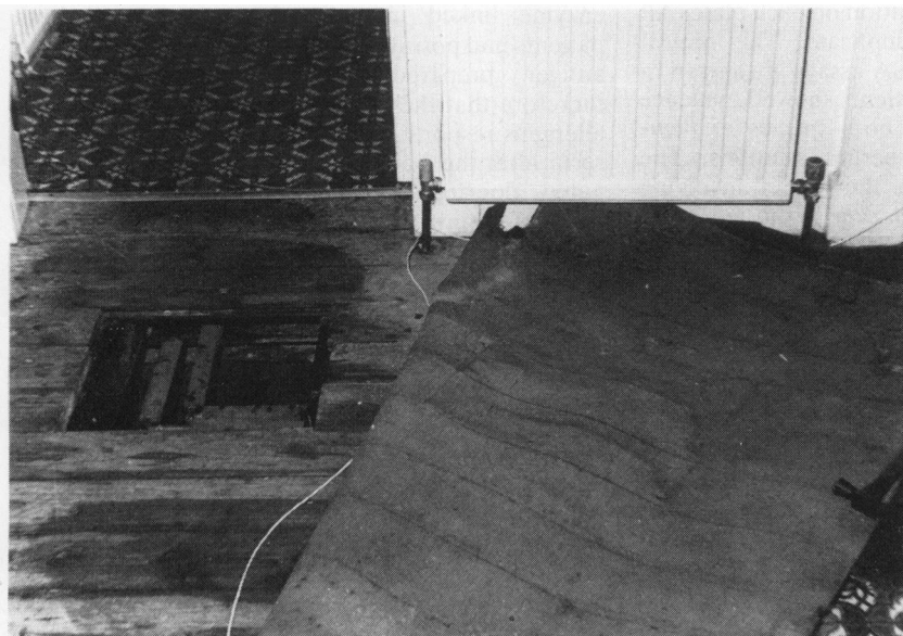
Fig 3 The patients' hall with wet flooring and mouldy linoleum (photograph taken 24 hours after the leak was discovered).
