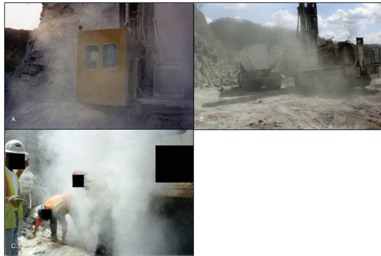
FIGURE 4. Photographs taken at the worksite by Miner 8. (A) Taken in 1981 at a surface coal mine, it shows a dust cloud enveloping the operator's cab on a surface drill. (B) Taken in 2010 at a surface coal mine, it shows a cloud of dust around an Ingersoll Rand 45 drill and a worker to the left of the haul truck. (C) Taken in 2012 at a surface coal mine, it shows three miners enveloped in a dust cloud loading drill holes to blast overburden.
