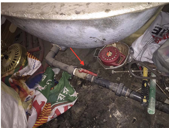
Figure 2 An inspection revealed an unhygienic storage area with leaky connection points to the consumer access point. Arrows indicate water leaking from pipes.
