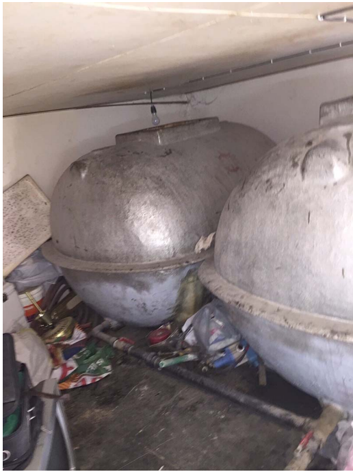
Figure 1 The two tanks used to store water from the desalination plant.
