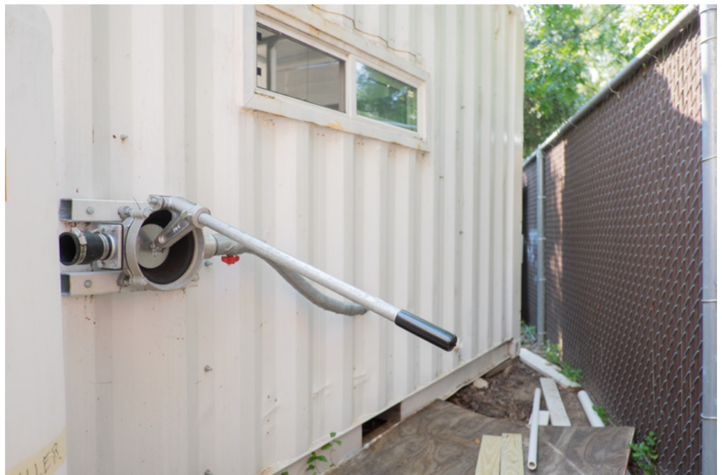
Fig 3. Water tank and hand-powered pump.
