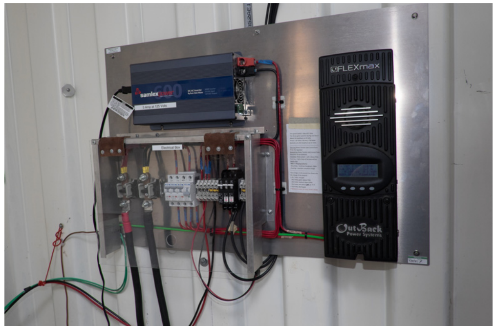
Fig 7. Electrical control plate inside of container.
