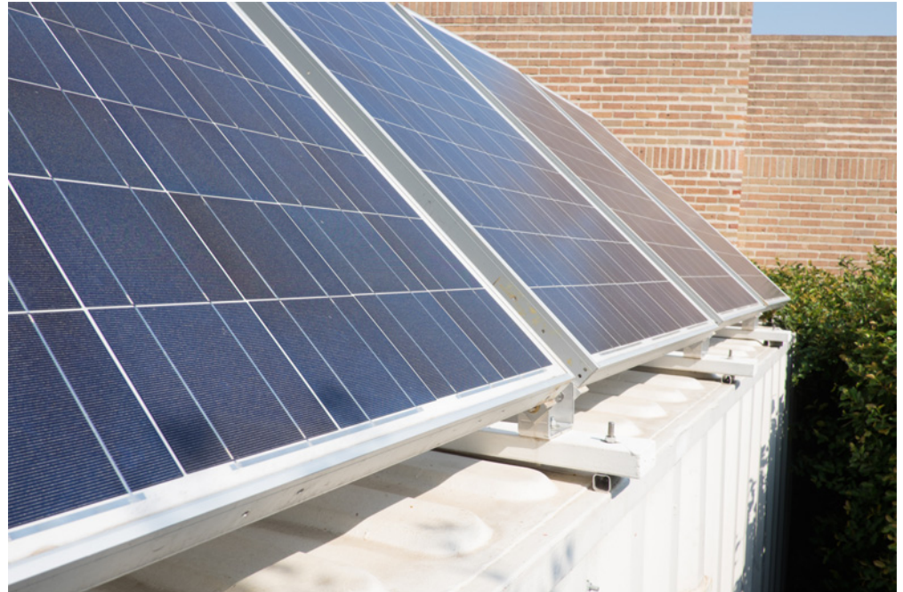
Fig 6. Solar PV panels mounted on container's roof.
