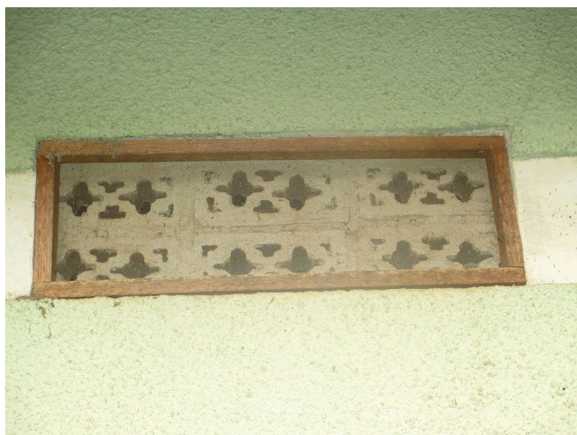
Fig. 1 A ventilator with screening on one of the demonstration houses
