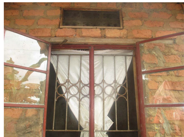
Fig. 3 A window and ventilator with screening on one of the demonstration houses
