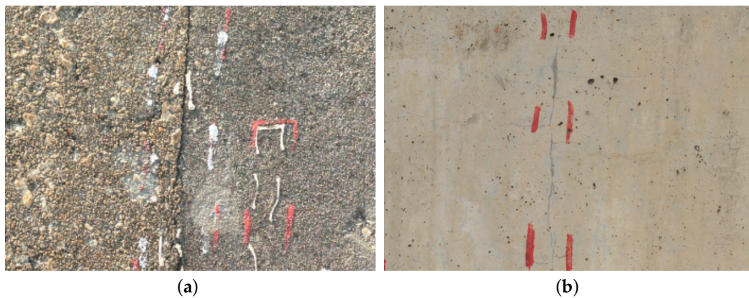
Figure 5. The geometry of cracks on the surface of RCB. (a) Crack shape one; (b) Crack shape two.
