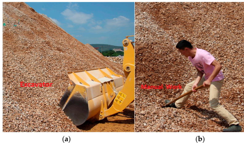
Figure 12. (a) Digging out the slope with an excavator; (b) Manually digging out the slope.
