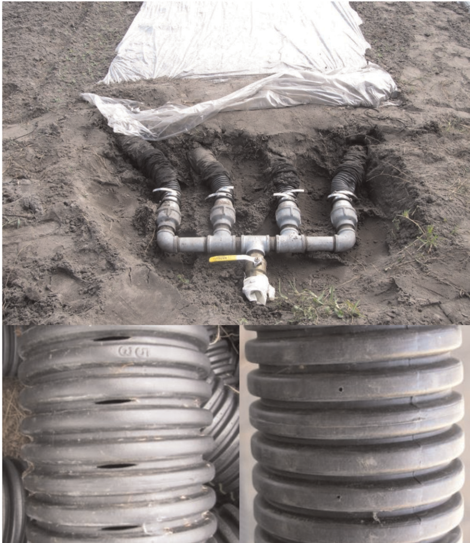
FIG. 1. Perforated medium density polyethylene plastic pipe (7.6 cm diameter) used with saturated steam. This method is well suited for combined use with solarization, and is relatively efficient with regard to fuel consumption. Four pipes were installed in each planting bed, with at least one pipe per foot of bed width. Pipes were laid in trenches at 35-cm depth with the objective of heating the top 20 cm of soil. Lower right: standard 7.6 cm perforated plastic drain tile (steam 1), lower left: custom-drilled plastic drain tile with 1.6-mm holes spaced every 3.8 cm (steam 2).
