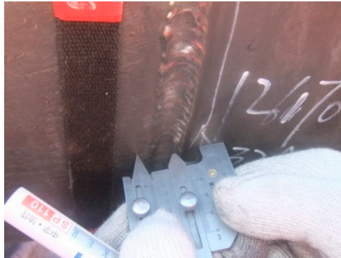
Figure 5. Profile of a mismatched weld joint.
