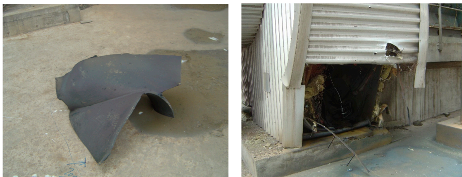
Figure 17. Photograph of destroyed housing of the BFG booster.
