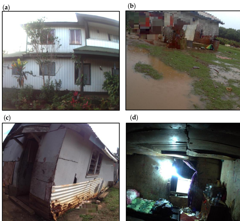
Figure 1. Range of house quality observed: (a) House without any evidence of structural damage and exterior is well maintained; (b) House surrounded by pools of rain water due to insufficient drainage, interior of house water damaged; (c) Poor building quality indicated by holes in the external wall and use of building materials to patch up exterior; (d) Children’s bedroom with damaged ceiling and walls, and evidence of water staining on the cardboard covering holes in the ceiling.
