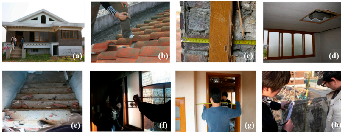
Figure 1. Taking measurements of building characteristics at different locations: (a) surveying general characteristics of a building; (b) roof; (c) wall; (d) floor and ceiling; (e) stairs; (f) windows; (g) door; and, (h) wall/fence.
