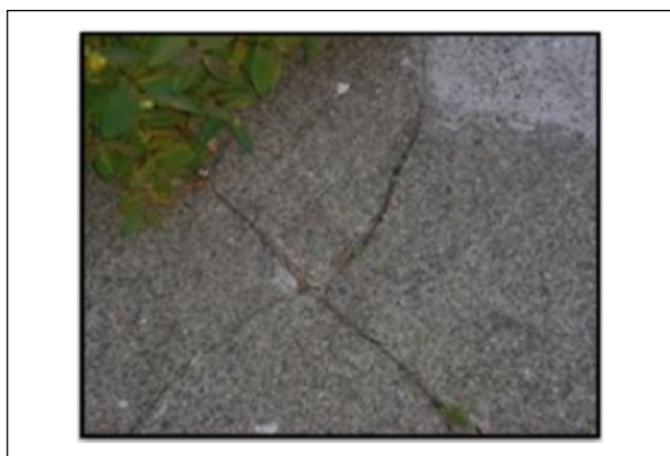
Figure 4. Cracks in the Concrete.
