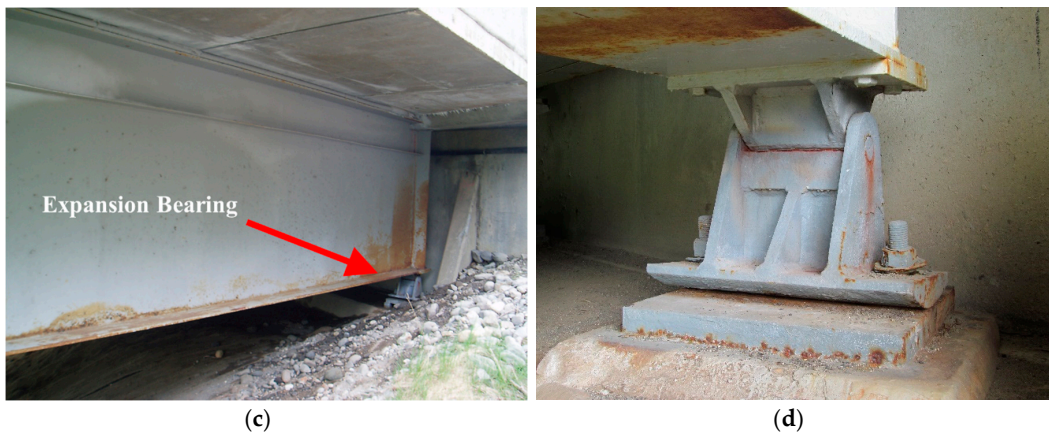
Figure 1. Photographs: (a) Chulitna River Bridge; (b) Bridge bottom view; (c) Expansion bearing at the bridge end; (d) Expansion bearing.
