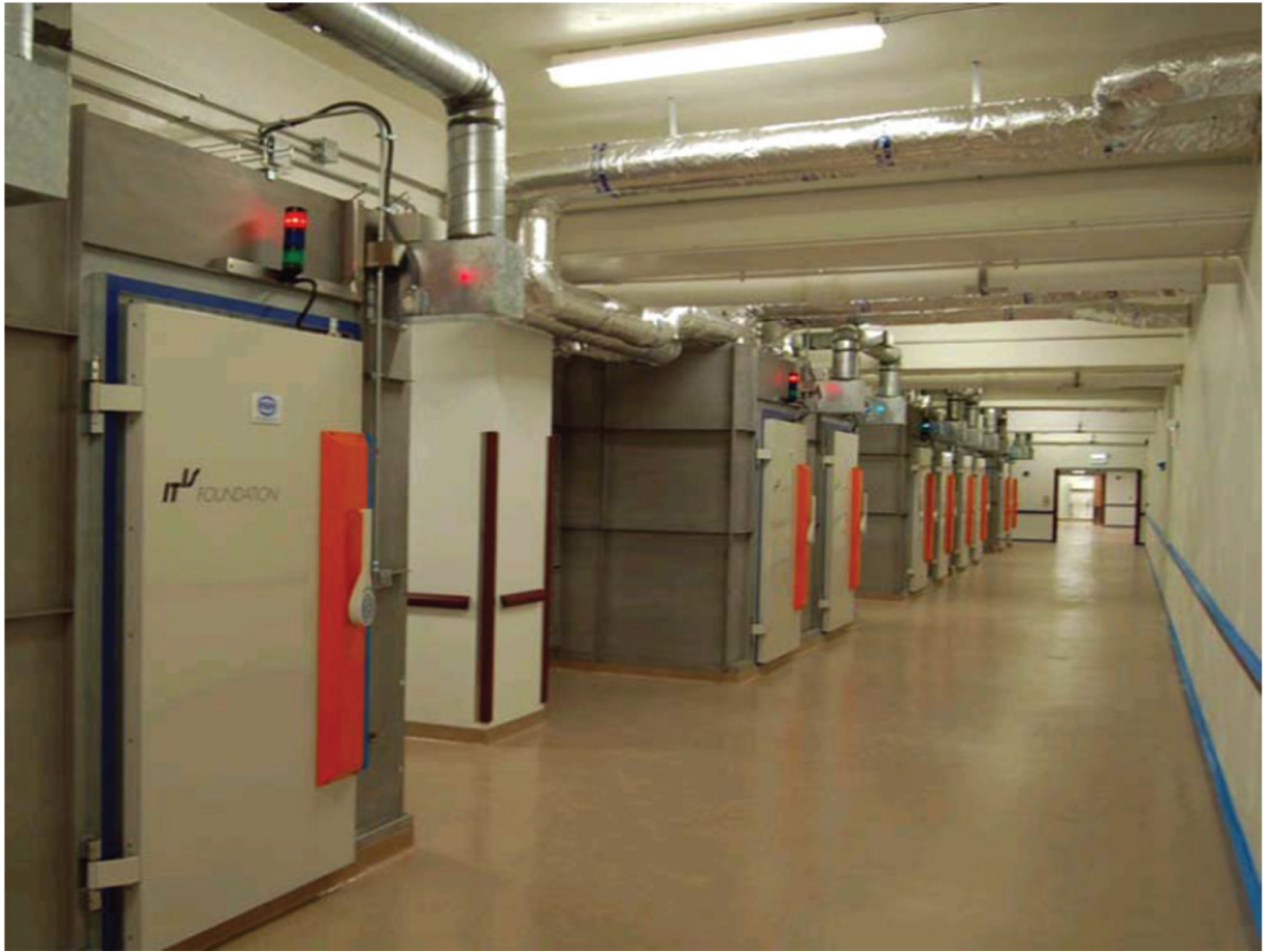
Fig. 5. RFR reverberation chambers installed at IITRI.
