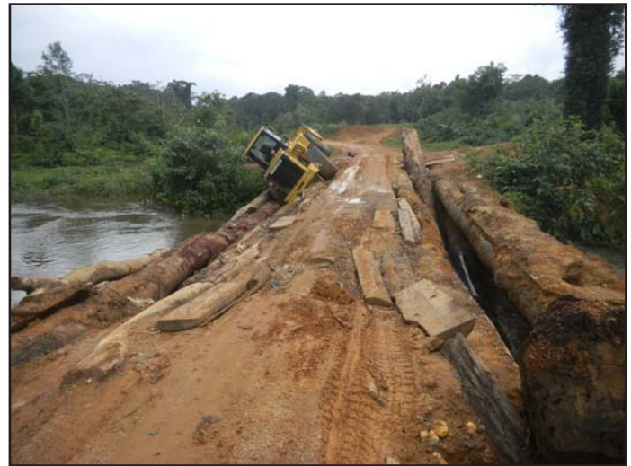
FIGURE 3. A nearly impassable bridge on the road connecting Sinoe County with Monrovia, the closest location with Ebola treatment units — Liberia, September 2014
