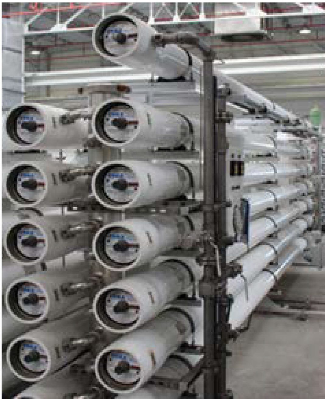
Figure 11. Spiral wound RO membranes installed in Groundwater Replenishment System (GWRS) Advanced Water Purification Facility (Fountain Valley, California), taken at the Orange County Water District.
