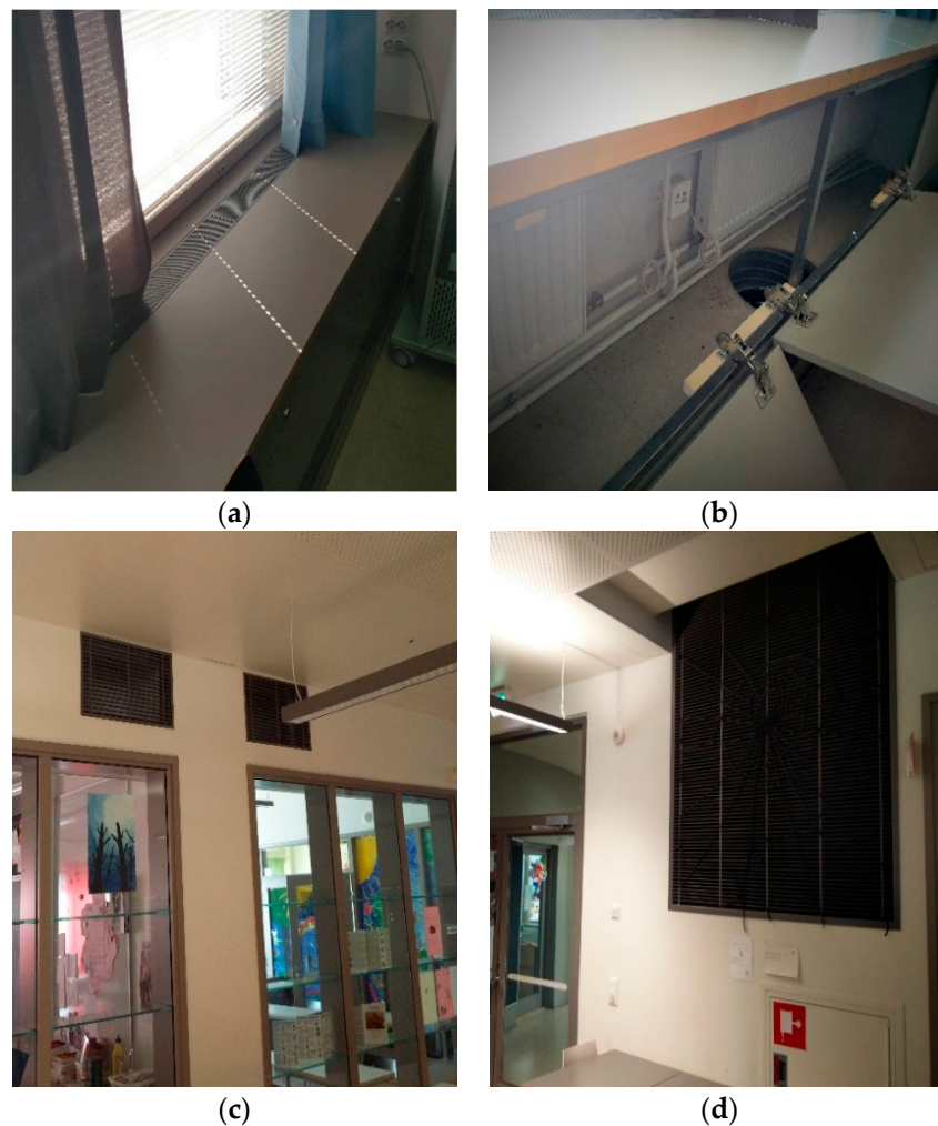
Figure 3. (a,b) Supply air grill and duct in the classrooms; (c) transfer air grilles in the partitions between classrooms and the lobby and (d) exhaust stack in the lobby.
