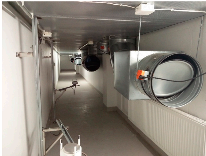
Figure 4. Supply air duct corridor and classroom-specific ducts' terminal units in the basement. Dampers are opened 20%, as designed.
