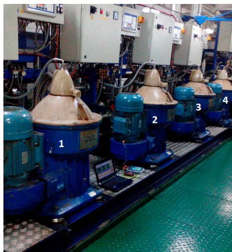
Figure 1. Photography of four marine oil Separators Alfa Laval SA 831 labeled with their corresponding numbers.
