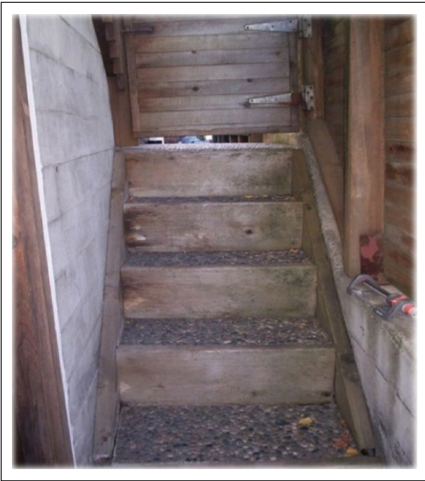
Figure 2. The stairs the participant used to carry his yard tools to the front yard.
