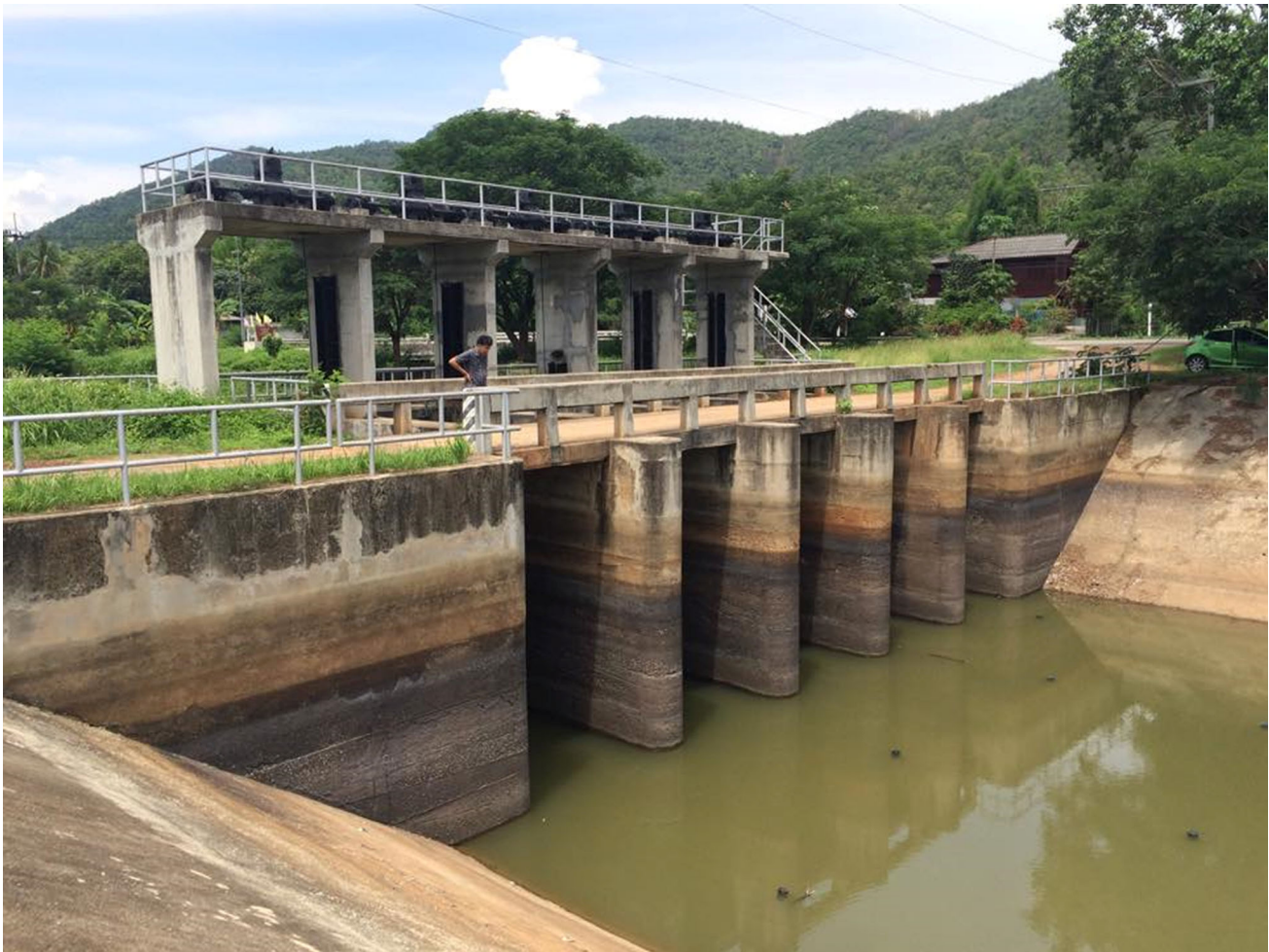
Fig. 3 Dam construction viewed from upstream, looking downstream, showing the low water level in the reservoir. Source Author's photo
