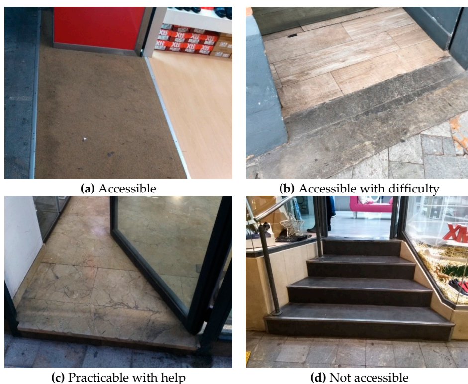
Figure 2. Samples of the four levels of accessibility found in the field study. (a) A store with accessible entrance. (b) An entrance accessible with some difficulty. (c) An entrance that can be accessed with the help of other people. (d) A not accessible entrance.
