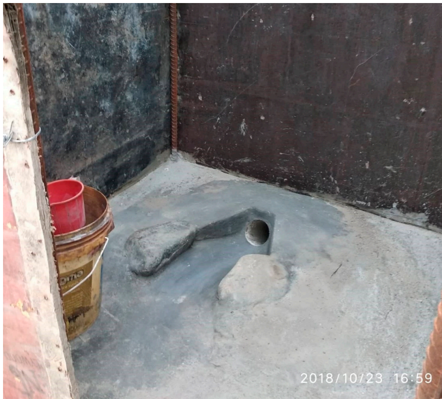
Figure 2. Example of a low-cost improved sanitation facility in a construction site. Photo credit: Sudeep Sharma.
