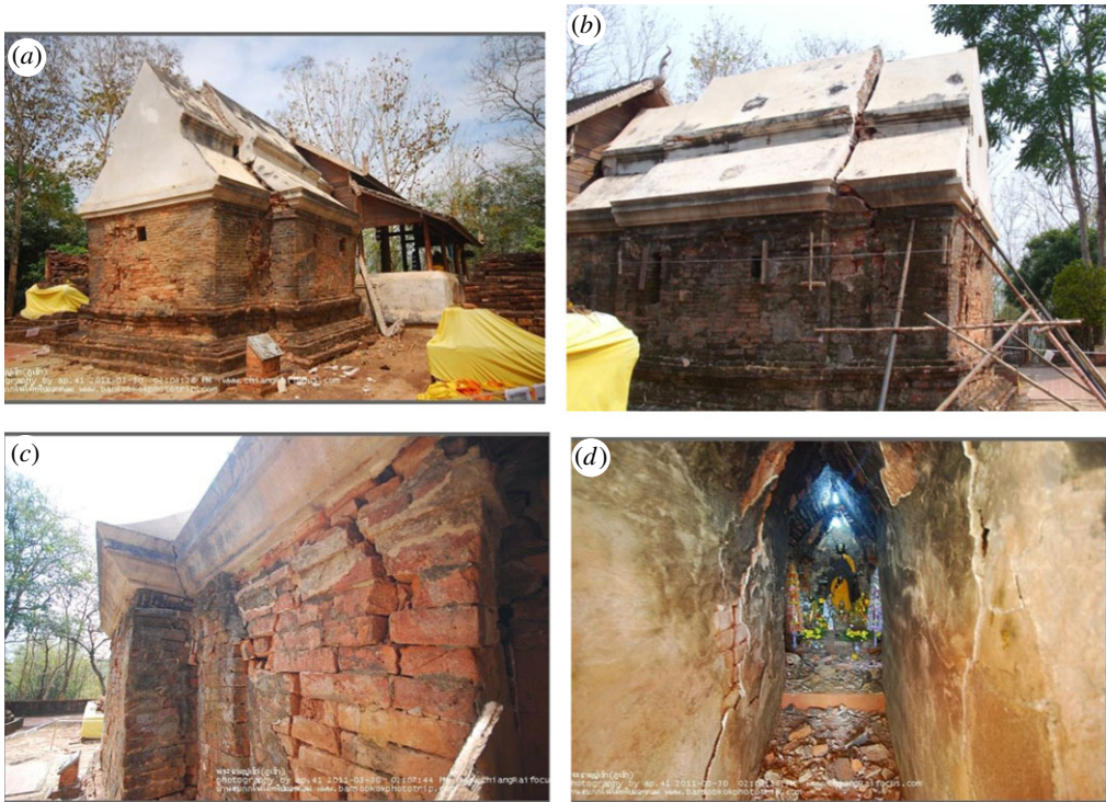
Figure 6. (a) Pu Khao temple damage due to 2011 earthquake viewed from NE. (b) The same photograph viewed from SW. (c) Observed wide cracks at exterior walls. (d) Diagonal in-plane shear cracks could be clearly seen. (Online version in colour.)
