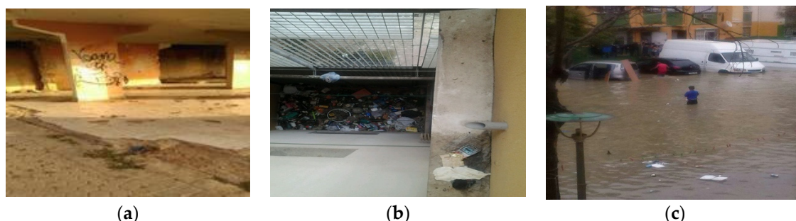
Figure 5. Unlivable housing conditions. (a) “There was a rehabilitation plan, they took the people out for construction and it was left half done”. Despite local rehabilitation plans, “These buildings have been like this for ten years . . . homeless people and drug addicts occupy the building . . . when they are cold they build fireplaces and the building goes up in flames constantly”. (b) “There is a hole where a wash sink was that was torn out and now it is full of trash. Next door there are people who live with the trash and smell”. (c) This was a photograph a neighbor sent to the Whatsapp group after we finished the formal Photovoice sessions. After a day of rainfall in Sevilla, neighbors were unable to leave their homes because of the poor sewage system.
