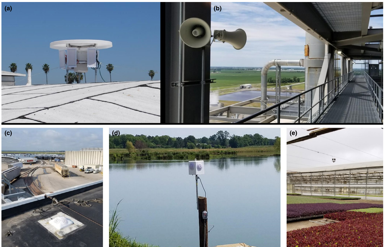
FIGURE 1 These images show some of the commercial installations of SonicNets. These installations include a directional system installed on the roof of a strip mall (a), a custom system in the superstructure of a coal power plant (b), an omnidirectional system installed on the roof of a meat processing plant (c), an omnidirectional system installed at a catfish farm (d), and an omnidirectional system installed in a plant nursery (e). Each of these systems were successful at deterring the birds from the targeted region, but there is only qualitative and anecdotal data. All images were provided by Midstream Technology
