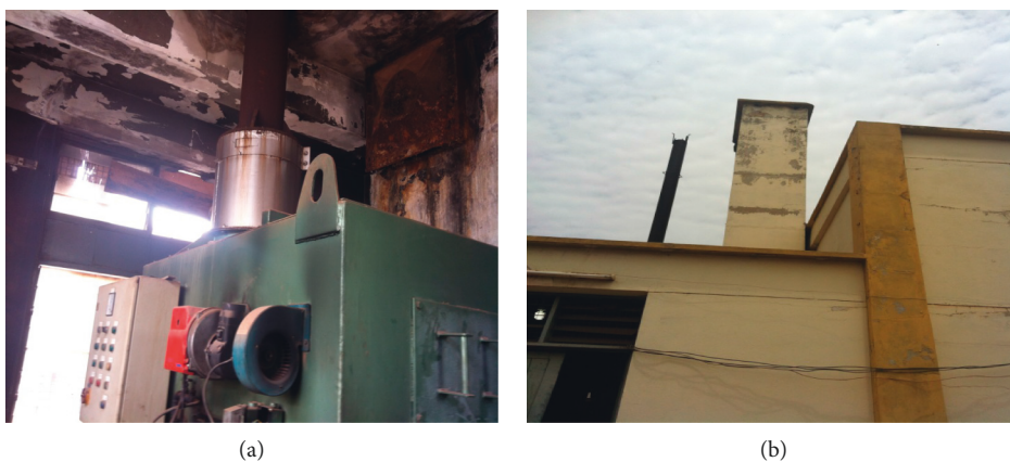
FIGURE 13: Anatomic waste incinerator at KATH. (a) Combustion chamber. (b) Chimney.
