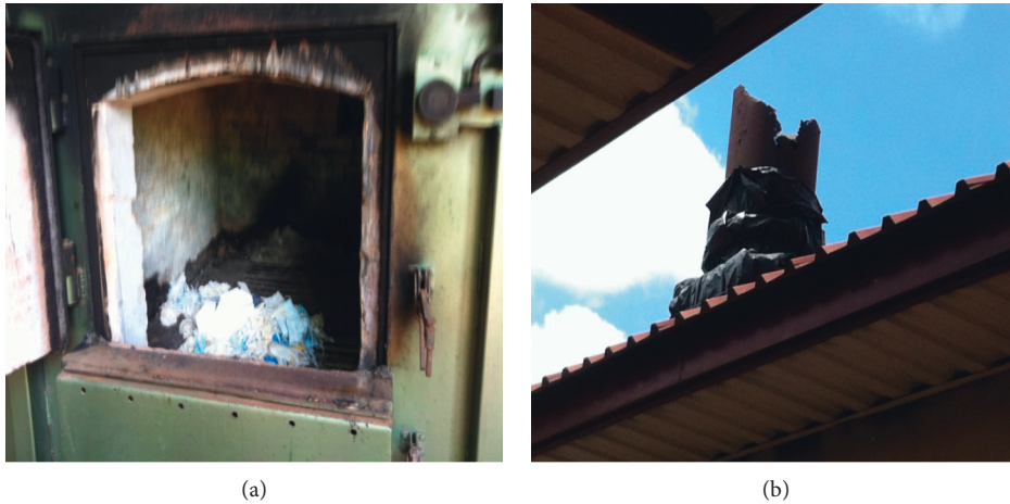
FIGURE 11: Imported incinerator at Brong Regional Hospital, Sunyani. (a) Combustion chamber. (b) Chimney without APCD.
