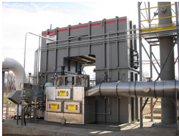
Figure 3.27 Regenerative thermal oxidizer, photograph.
