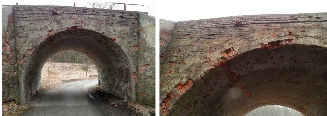
Figure 1. Side view of masonry arch viaduct before restoration: (a) Overview, (b) visible damage (deflection from the vertical) of the parapet (upper part of the headwall), which was caused by the root.
