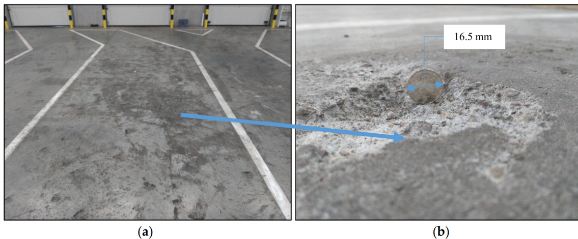
Figure 1. Example of crumbling on the top layer of concrete industrial floor: (a) General view; (b) close-up of cracked surface.
