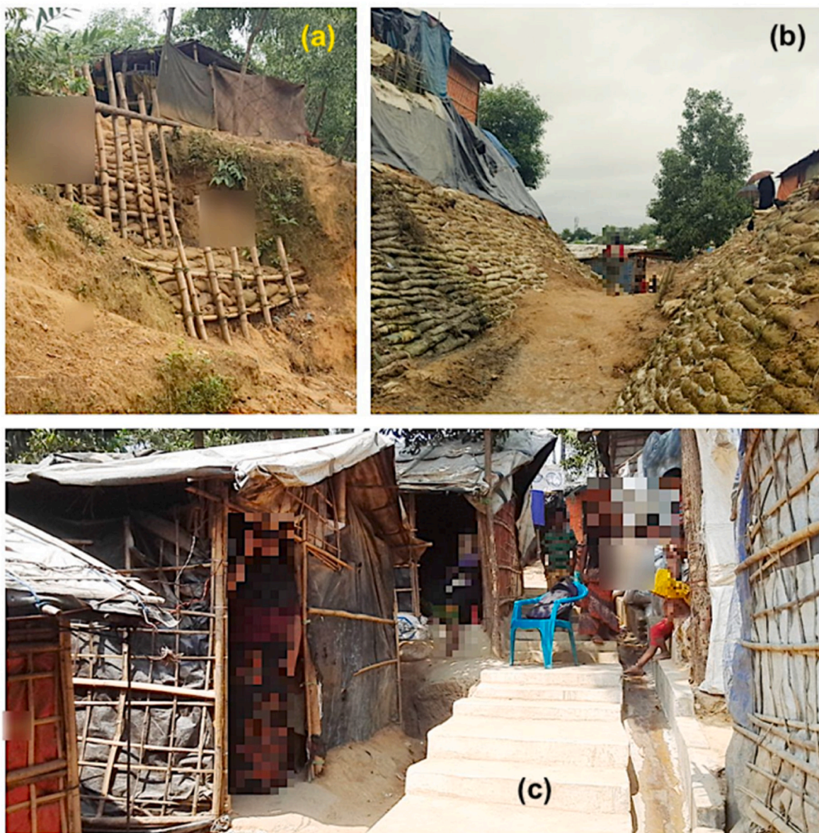
Fig. 8. Ongoing site development works (a) placement of bamboos, (b) sandbags to stabilise hill slope, and (c) construction of drainage system to channelize the flow of rainwater (Source: Fieldwork, May 2019).
