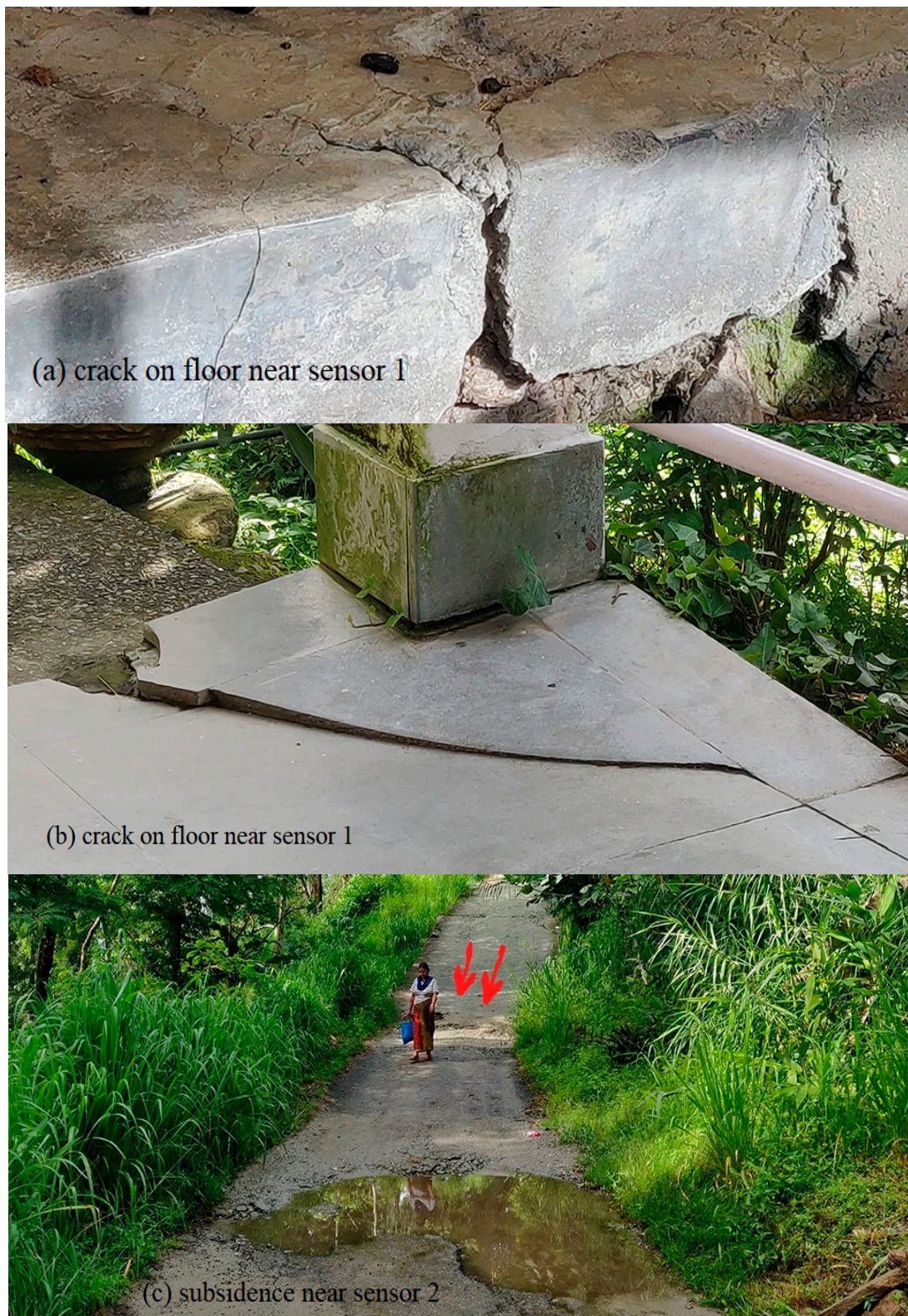
Figure 13. Displacements observed after the 2019 monsoon: (a) crack on floor near sensor 1, (b) crack on floor near sensor 1, (c) subsidence near sensor 2.
