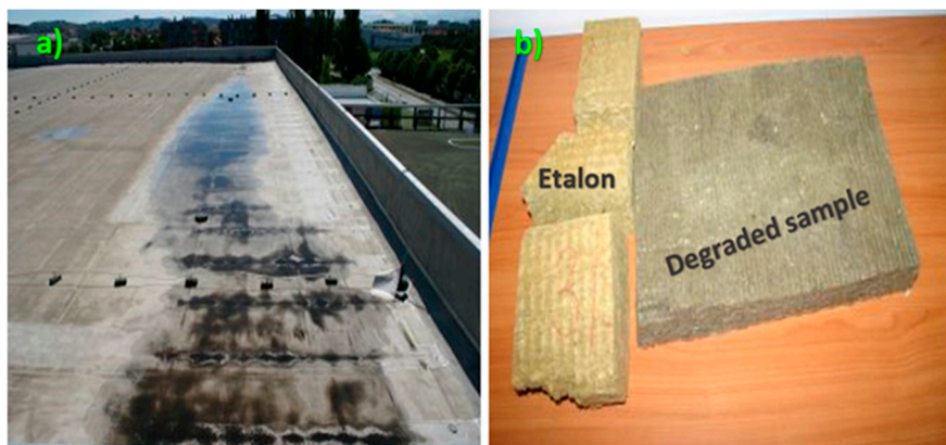
Figure 2. (a) Mineral wool samples taken from softened, uneven roofing areas of a commercial building located in Slovenia, Central Europe. (b) Visual presentation of new and degraded insulation samples.
