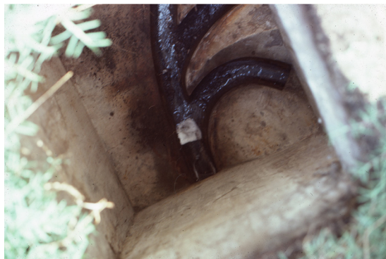
FIG 4 Sewer swab placed in the small diameter sewer draining three households in Santiago, Chile, in January 1983.
