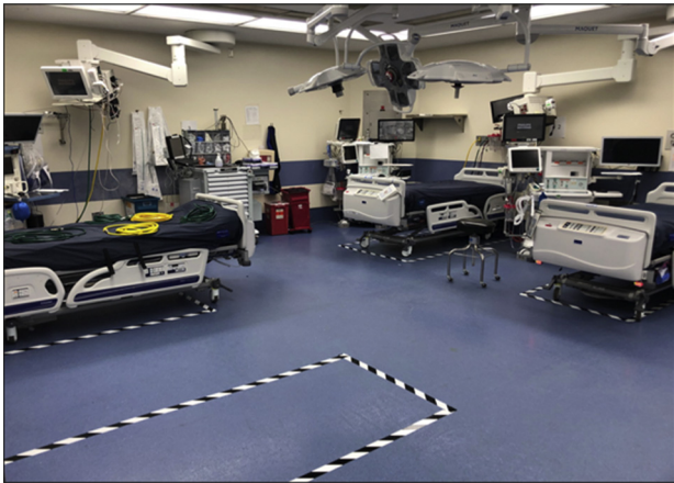
FIGURE 1. Representative photograph of an ORICU: This is an operating room that has been modified to accommodate up to 4 ventilated patients with COVID-19, each with a separate ventilator, gas lines, and other equipment.
