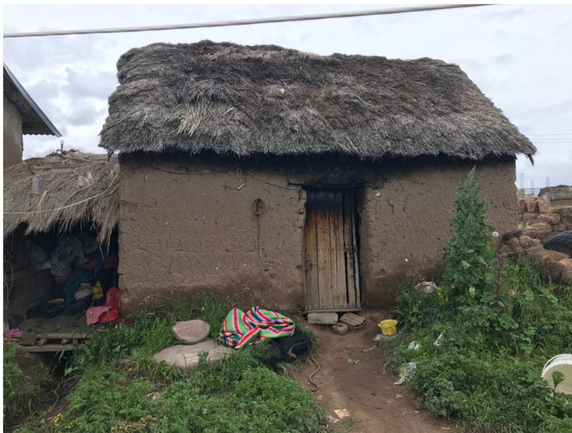
Figure 2. Adobe kitchen structure with thatch roof common in Puno. Some households have aluminum roofs.
