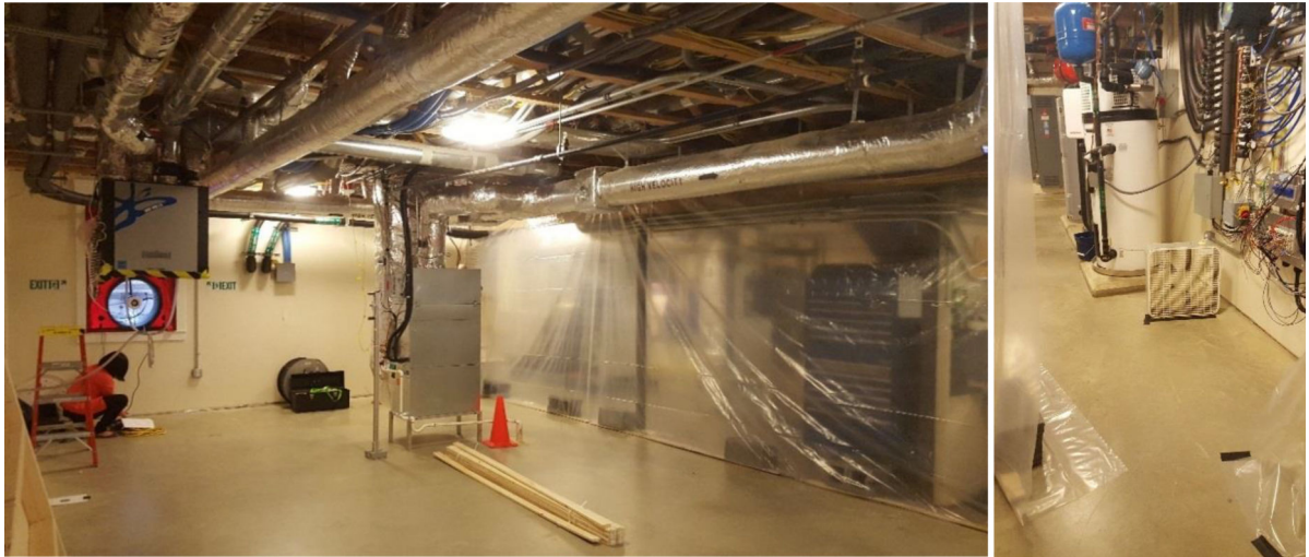
Figure 3. Photograph of the isolation area formed with poly polyethylene sheet and blower door fan in the window well (Left). Photograph of the directing fan and access area to the isolation area (Right).
