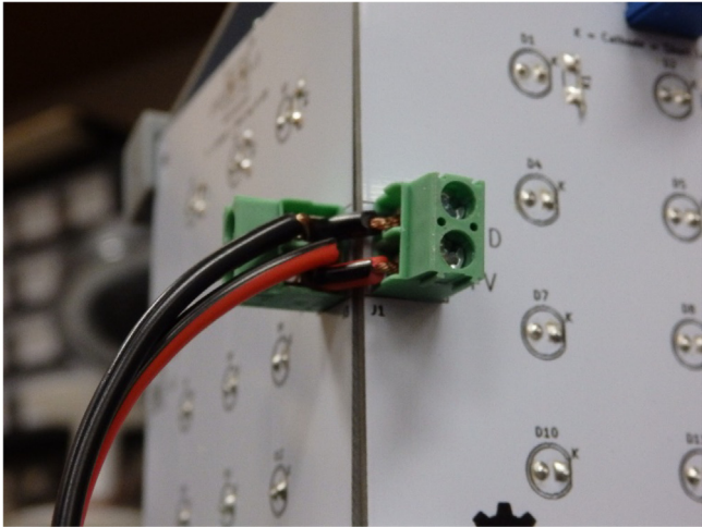
Fig. 11. Two cables tapped into a terminal set for power flow from the supply.
