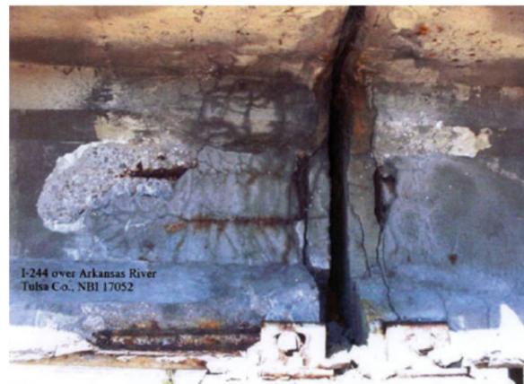
Figure 12. Damage in the end region of an AASHTO bridge girder [21].
