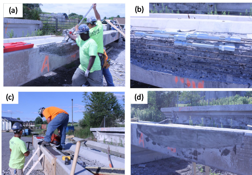
Figure 11. Repair procedure using strand splices: (a) installation of the strand splices, (b) completed installation of splices, (c) placing the repair concrete, and (d) completed repair after form removal (adopted from [19]).
