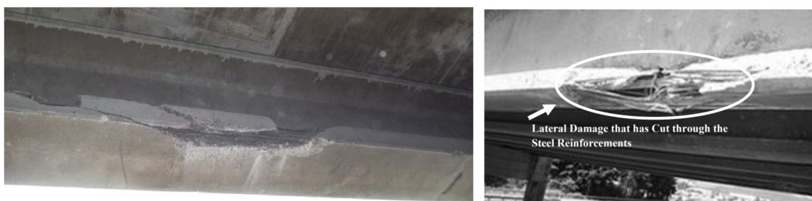
Figure 19. Severe concrete spalling due to overheight truck impact damage [6], and example of lateral impact damage on steel reinforcement [24].
