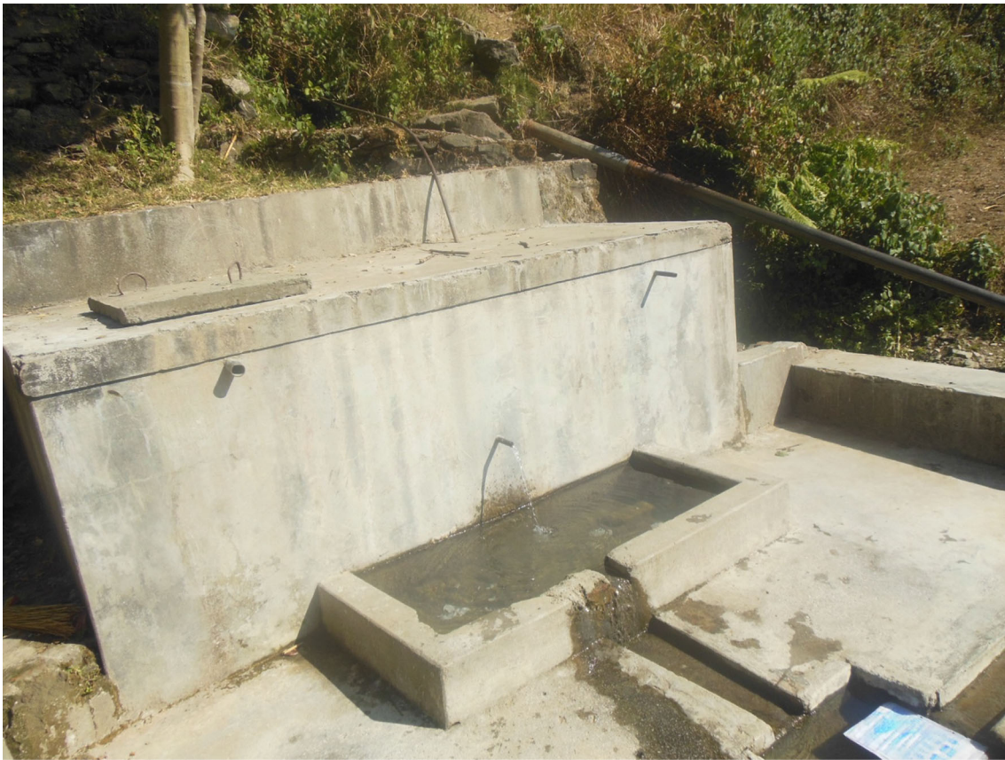
Fig. 4 Water tank built by PMC near Bohal Spring source. Photo by Anjali Uniyal
