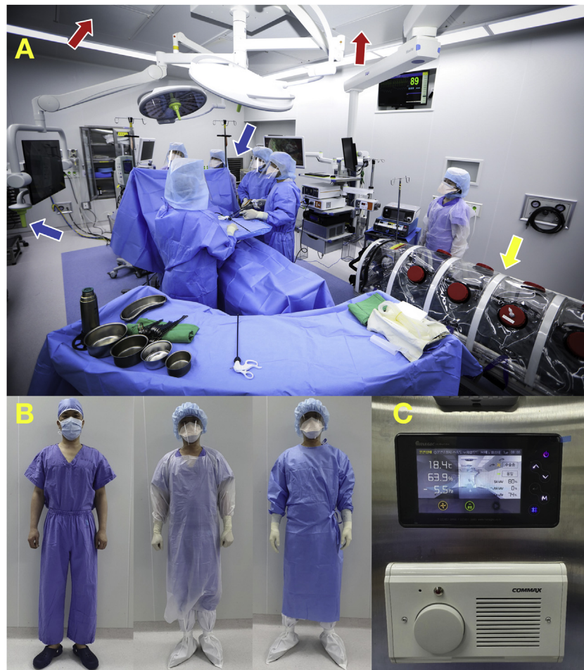
Fig. 2. A) View of the entire negative-pressure operating room. The surgical team is wearing enhanced personal protective equipment and a negative-pressure cart is shown (yellow arrow). Airflow was maintained from the ceiling perforated supply diffuser (red arrow) to the exhaust grille (blue arrow) installed at the bottom of the four corners of the operating room. B) Surgical suit, an isolation gown, and enhanced personal protective equipment. C) Negative-pressure status display panel and intercom installed outside the entrance of the negative-pressure operating room.
