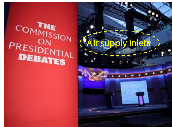
FIG. 2. Air supply inlets installed above the debate stage.
