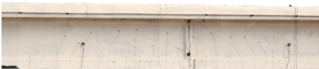
Figure 11. Visible cracks on girder T1 opened during the loading phase P3 4800 kN.
