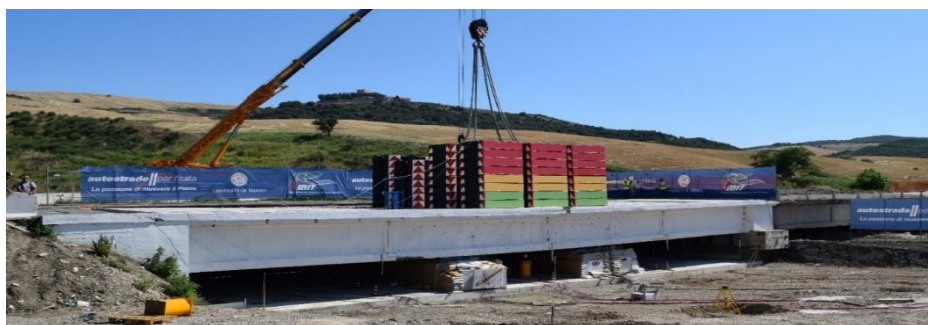
Figure 8. The Alveo Vecchio viaduct during the loading phase 5, loaded with 93 weights—9300 kN.
