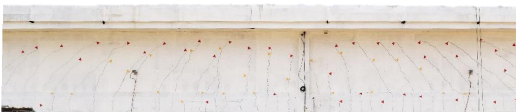
Figure 12. Visible cracks on girder T1 opened during the loading phase P4 7200 kN.
