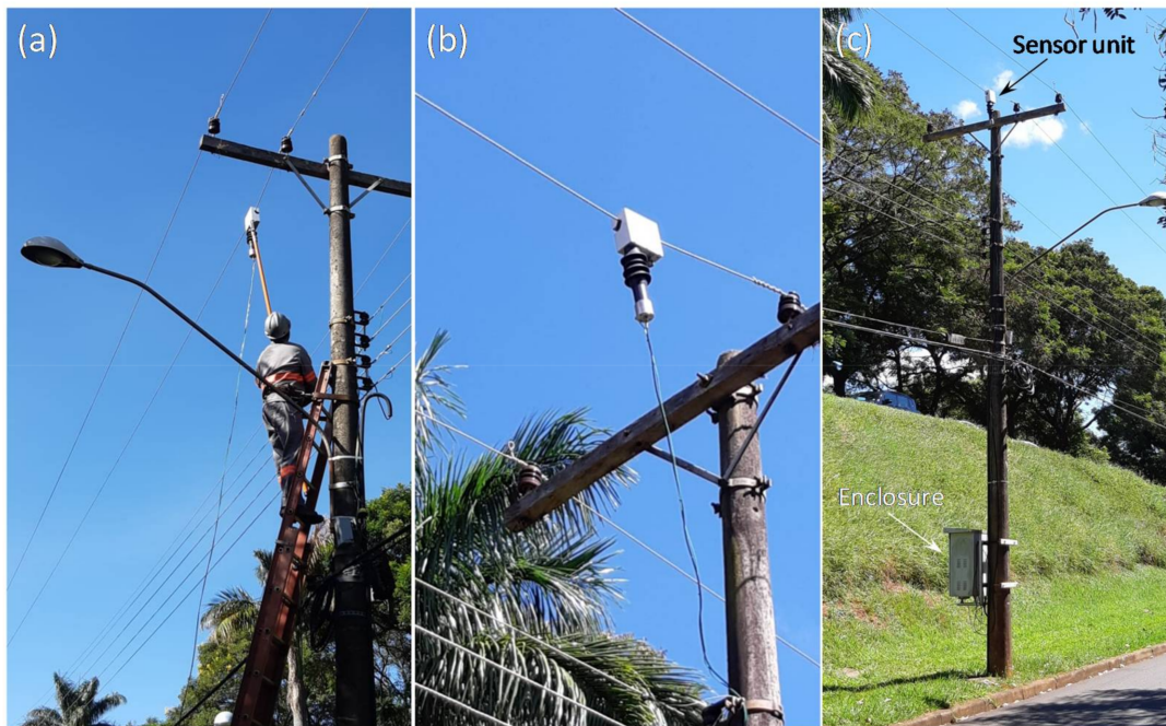
Figure A1. (a) Sensor installation in a phase of 11.9 kV distribution network, (b) sensor installed, and (c) the sensor and processing unit.
