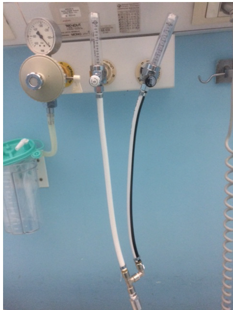
Figure 1. by means of a Y-shaped metal connector we built the connection between the oxygen openings, the compressed air openings and the corrugated pipe of the mask or of the NIV C-PAP hood; inside the Y it is possible to insert a joint that permits to supply oxygen by means of a Venturi mask or nasal prongs (when NIV is not necessary).
